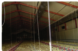
Poultry house using geothermal heating
