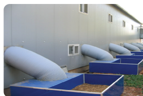
Offensive odor reducing device (open-type bio-filter system)
